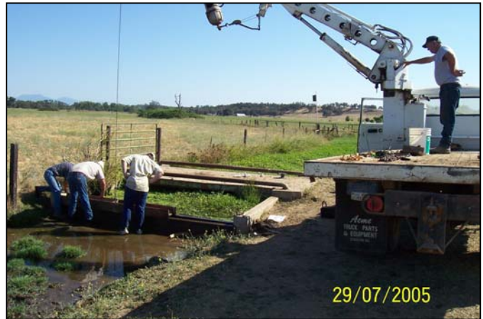
WC working landowners and the UCCE to install a tailwater retention pond release board.
