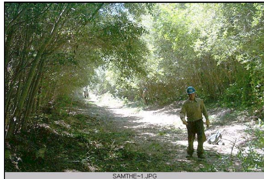
Completed clear and snag project. WC was instrumental in coordinating the project.
