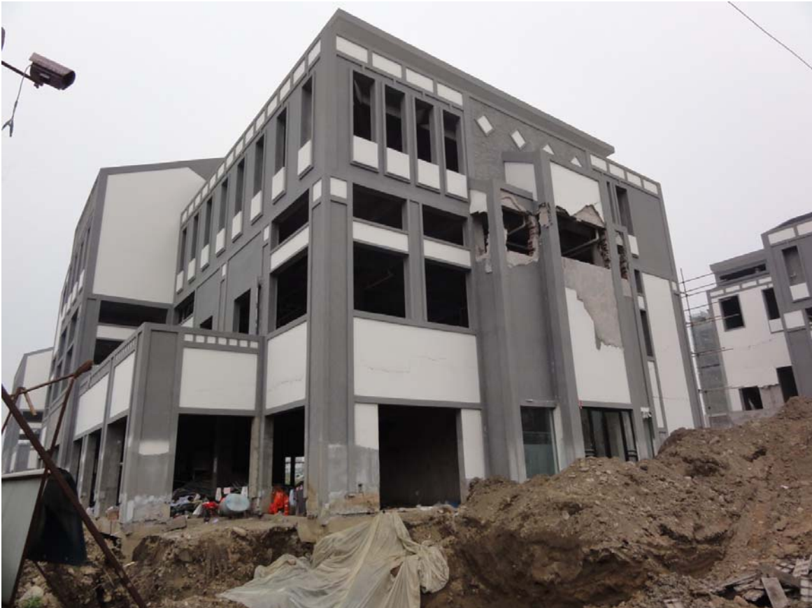
Fig. 16. New commercial building under construction with damage to brick infill.
