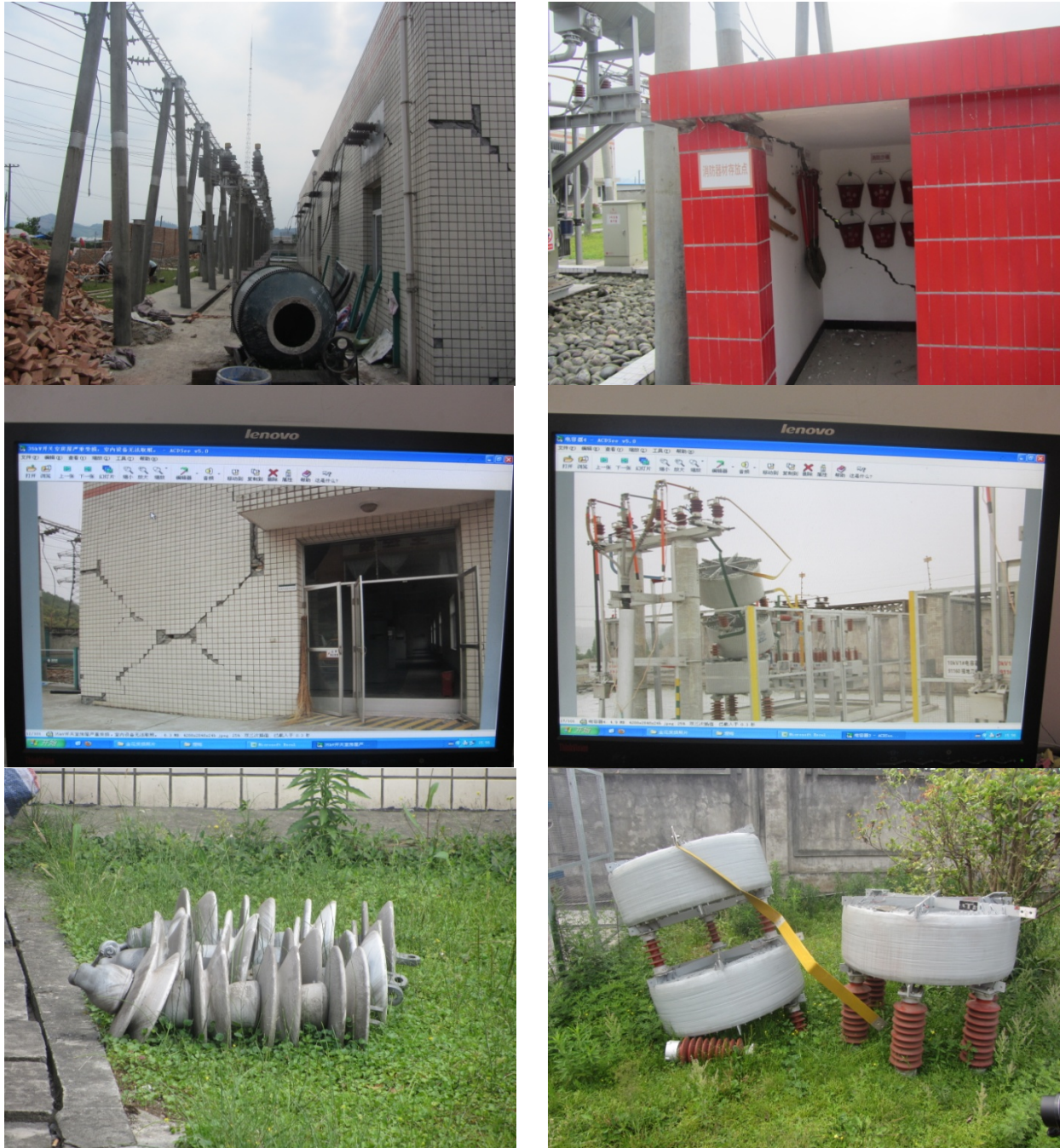
Fig. 22. Damage at the Jinhua 110kV Transformer Station. Photographs by Dr. Craig A. Davis.
