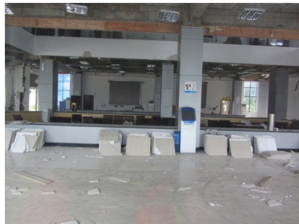
(d) Distress to ceiling tile and light fixtures; damage to non-structural walls. Photo by Dr. Craig A. Davis.
