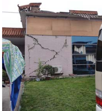
Fig. 8. Damage to Lushan County Government Building.
