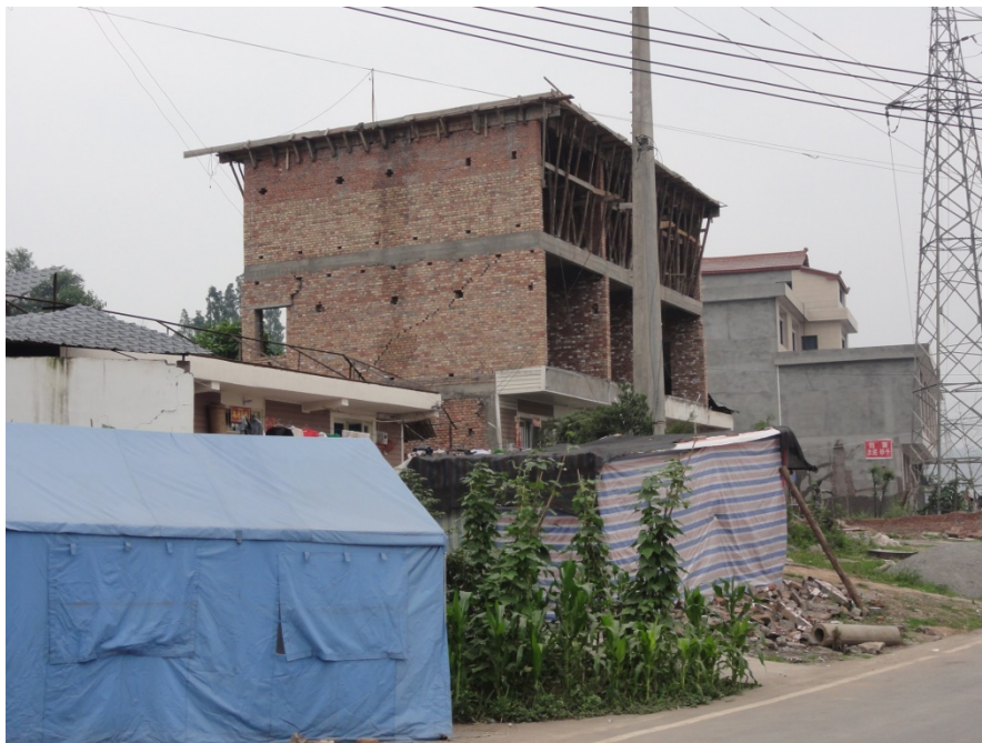
Fig. 12. Predominantly brick building without adequate reinforcement or confinement; note shear failures in wall at the second story.
