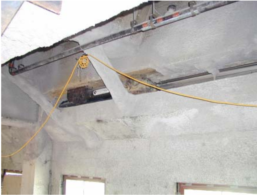
Figure 11: 225 kip damper installed at 26 th floor
