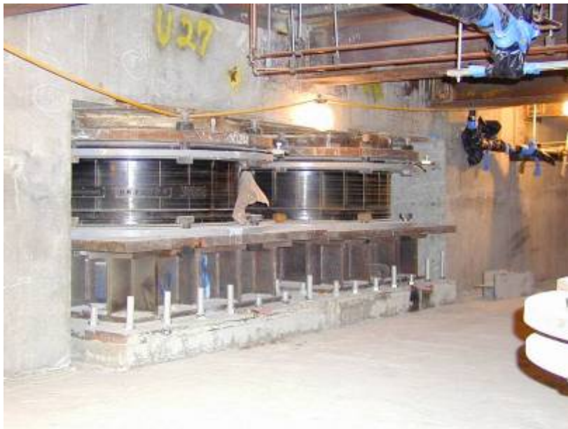
Figure 8: High damping rubber bearings installed under tower wall
