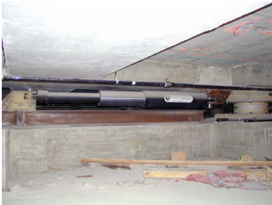
Figure 10: 300 kip damper installed at plane of isolation
