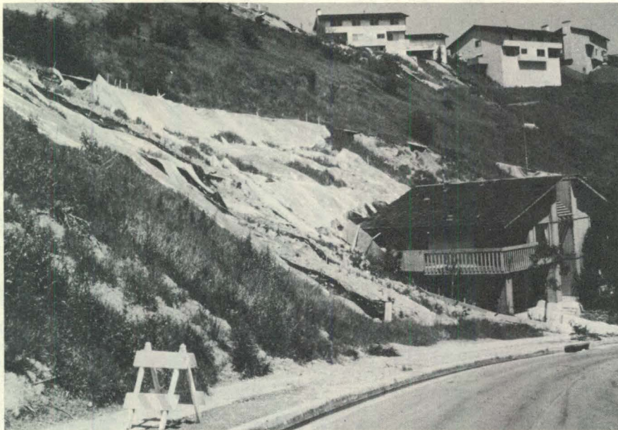
Hacienda Heights, Puente Hills; view southwest. Erosion and supersaturation of slopes beneath bench drains resulted in sloughing and debris flows which seriously damaged house in tract developed during 1970s. This was a widespread problem in this region.
