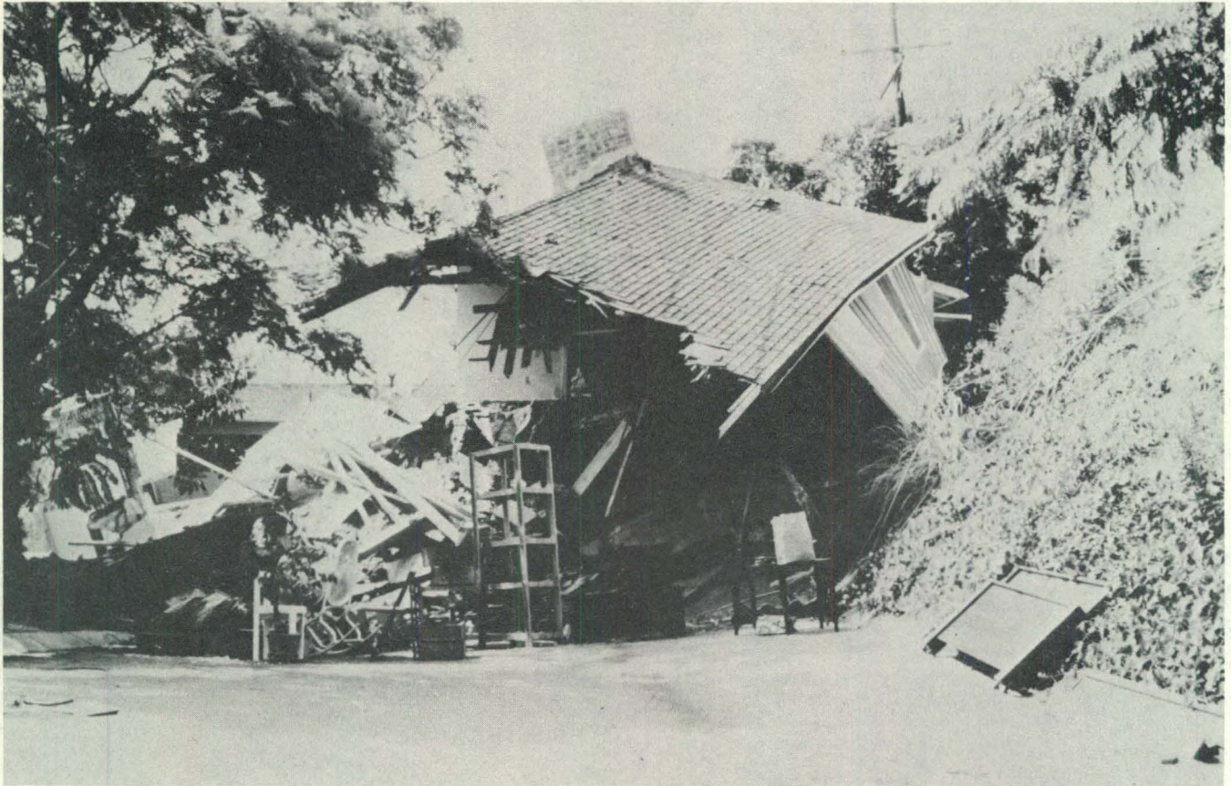
The Bluebird Canyon landslide damaged or destroyed more than 50 homes in a Laguna Beach hillside development. This house was destroyed when landslide movement began on October 2, 1978. For location of house, see upper left quadrant of lower left photo on front cover; see article, p. 5. Photo courtesy Slosson and Associates.
