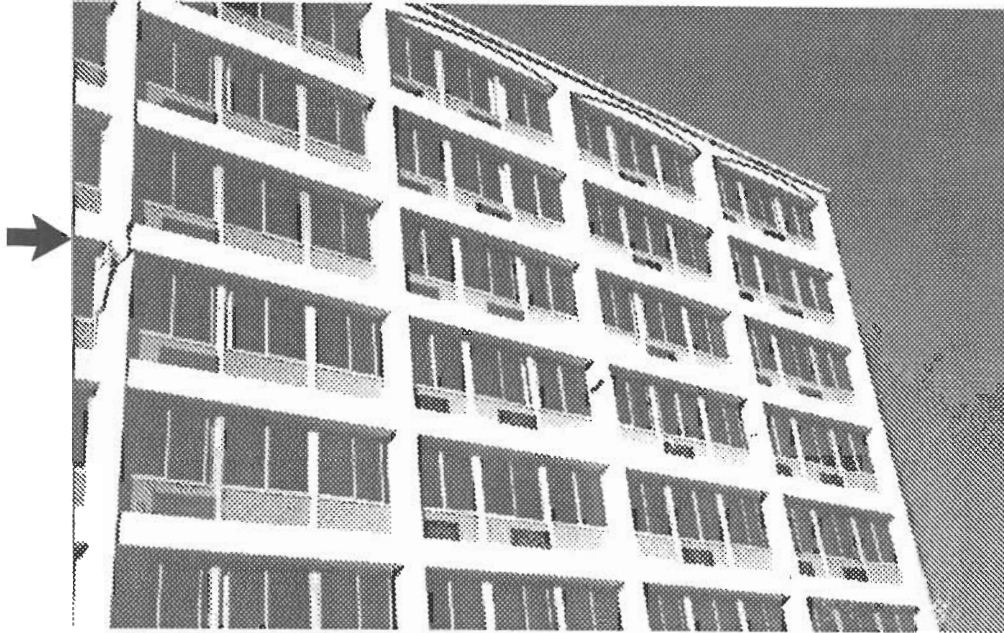
Fig. 5. Partial south elevation of Van Nuys 7-story Hotel showing damage to columns (indicated by an arrow) below fifth floor spandrel beams during the 1994 Northridge earthquake.
