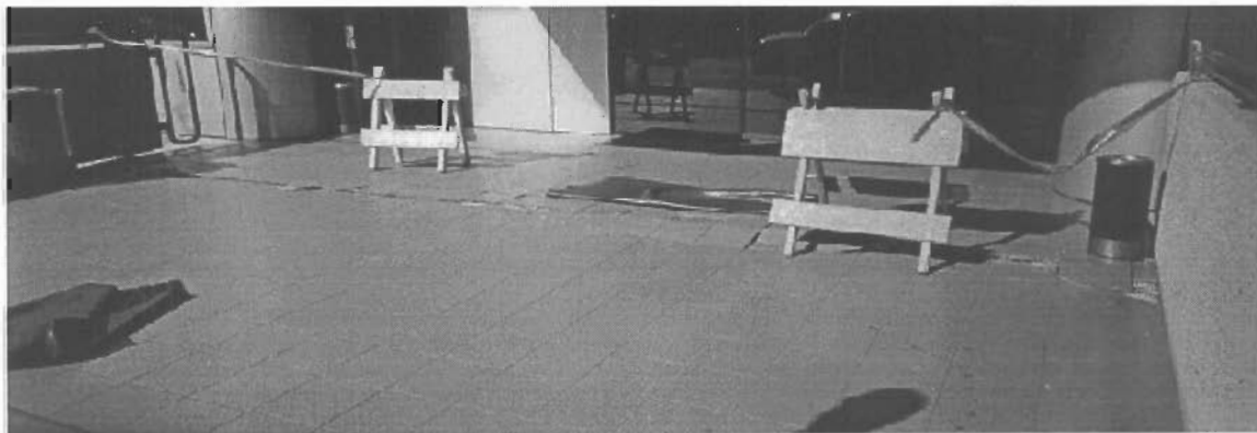
Figure 4. Tiles over isolation pit of the LACC 2 bldg. after the earthquake (photo courtesy of Robert Bachman).
