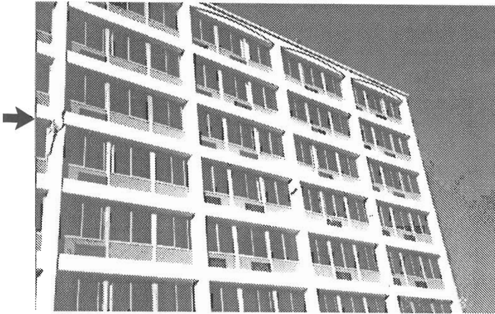
Fig. 5. Partial south elevation of Van Nuys 7-story Hotel showing damage to columns (indicated by an arrow) below fifth floor spandrel beams during the 1994 Northridge earthquake.
