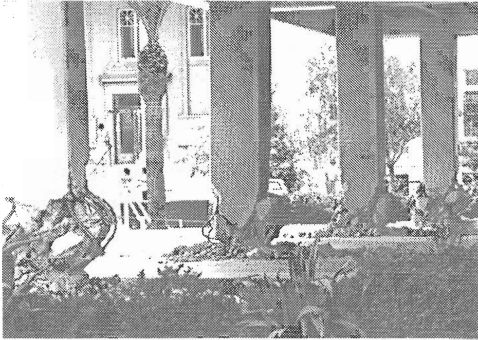
Fig. 1. Line of columns that failed at east end of the Imperial County Services Building during the 1979 Imperial Valley earthquake.
