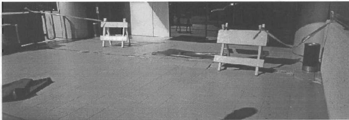
Figure 4. Tiles over isolation pit of the LACC 2 bldg. after the earthquake (photo courtesy of Robert Bachman).
