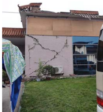
Fig. 8. Damage to Lushan County Government Building.
