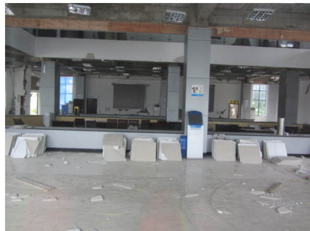
(d) Distress to ceiling tile and light fixtures; damage to non-structural walls. Photo by Dr. Craig A. Davis.
