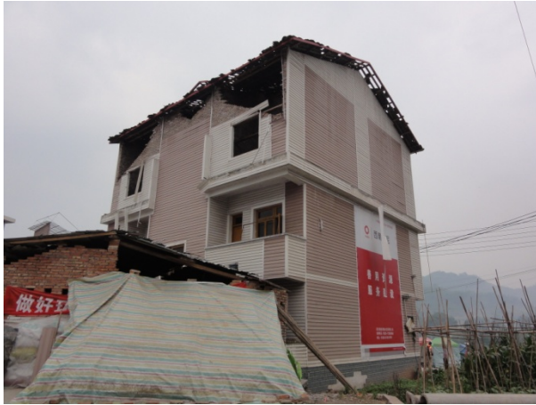
Fig. 10. Damaged residential building of brick construction.
