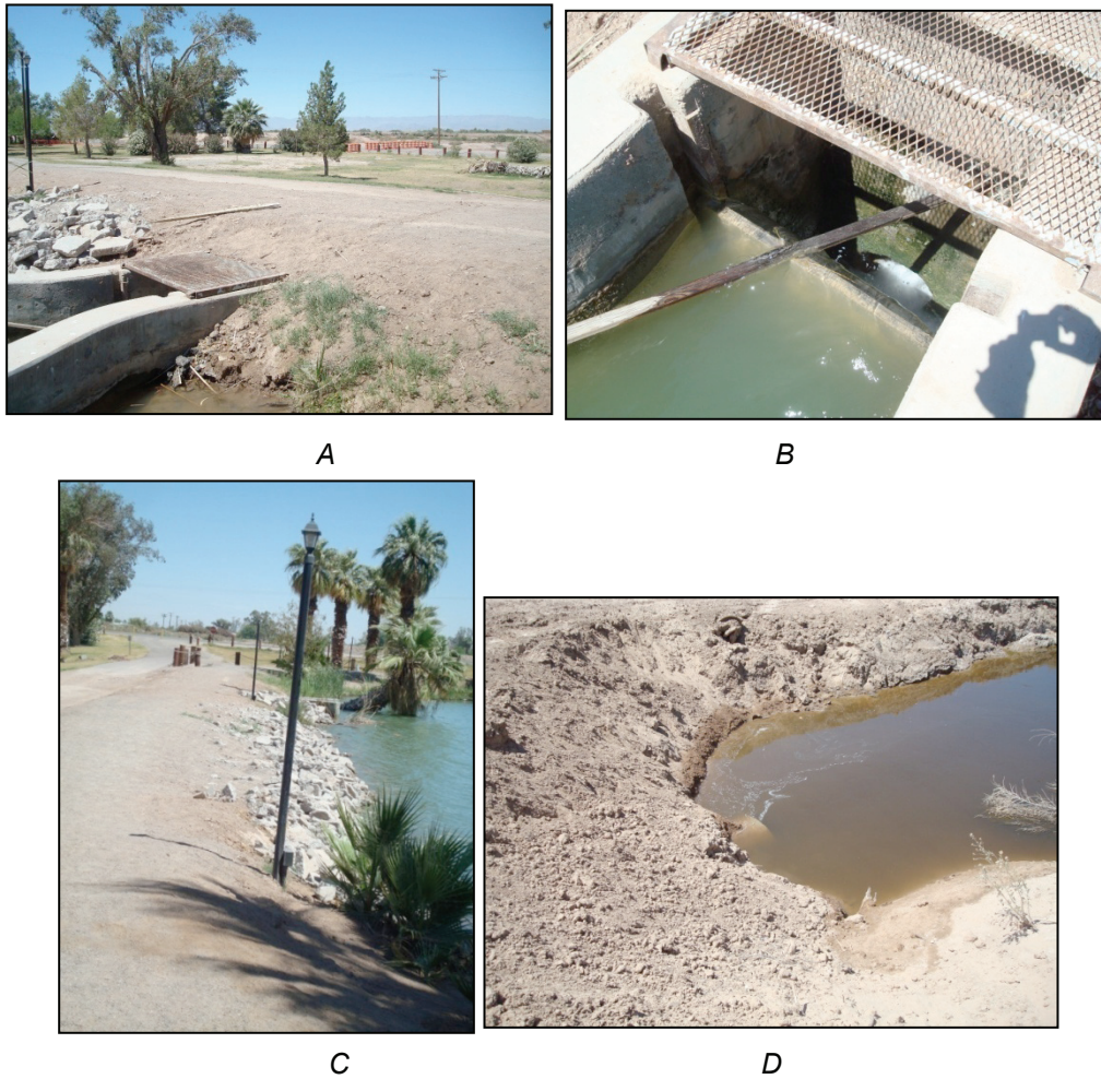
Figure 103. Repairs to Sunbeam Lake Dam and Drew Road as of June 8, 2010 (F02). A , Outlet weir and dam crest where sinkhole used to be. Note that barricades are still blocking Drew Road in the distance. B , View of water flowing over the weir and through the outlet pipe. C , Concrete rubble has been placed on the upstream side of the dam crest. Note that the lamp post is still leaning toward the lake as a result of the now-obsured lateral spreading. D , Repaired outlet pipe on the west side of Drew Road. Photos by T. McCrink, 6/8/10.
