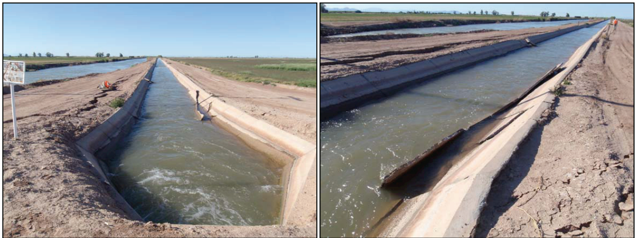
Figure 31. Images of Wormwood Canal flowing north from diversion from the All American Canal adjacent to Westside Main Canal (C01). The Westside Main Canal is visible to the west of Wormwood Canal. Lateral spreads on both sides of Wormwood Canal locally deformed the concrete liner, although the canal continued to function. Scarp height indicates about 14 cm of differential settlement. Photos by J. Tinsley, 4/6/10.
