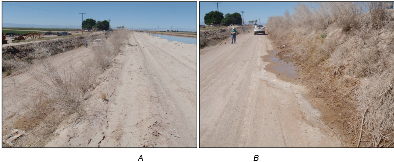
Figure 93. A, Overview of southeast levee confining the Westside Main Canal adjacent to Fites Road, showing minor extensional cracking at the outer edge (D15). Extensional cracking extended for a fraction of the length of the slope failure adjacent to the drainage channel at left. No vented liquefied materials were observed along the Westside Main Canal levee. B, View to southwest along Fites Road showing seepage from the Westside Main Canal, which created a puddle of standing water on Fites Road. Photos by J. Tinsley, 4/8/10.
