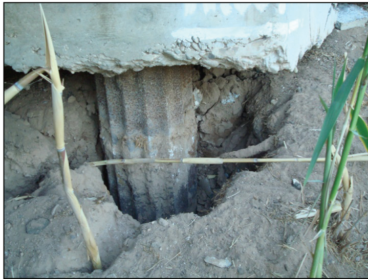
Figure 16. View of the concrete pier under the northeast corner of the Drew Road Bridge abutment (R07). Soil pushed away from the pier coupled with the battered asphalt on the road above (fig. 15) suggests that the bridge structure experienced large shaking displacements. Note spalled and cracked concrete in the abutment in the upper right corner of photograph. Photo by T. McCrink, 4/8/10.
