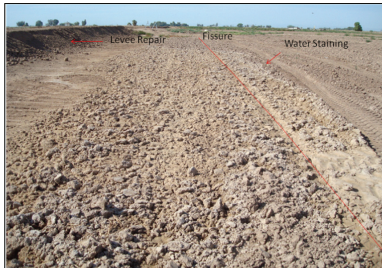
Figure 76. Evidence of excessive seepage from the east side of the Rosita Canal (C56). The fissure shown is slightly closer to the levee than the fissure related to the sand boils shown in figure 75. View to the north. Photo by T. McCrink, 4/11/10.
