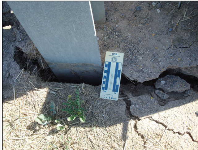
Figure 24. Bridge fill pushed away by the Worthington Road Bridge abutment due to strong shaking (R18). Photo by T. McCrink, 4/8/10.
