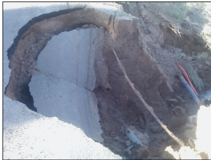
Figure 99. Close-up of the slump on the west side of Drew Road mentioned in the previous photo (R12). Several utility lines are exposed and some are broken. The outlet flow from Sunbeam Lake and probably the Seeley irrigation drain are just visible on the right. Photo courtesy of Imperial County Planning and Development Services Department.
