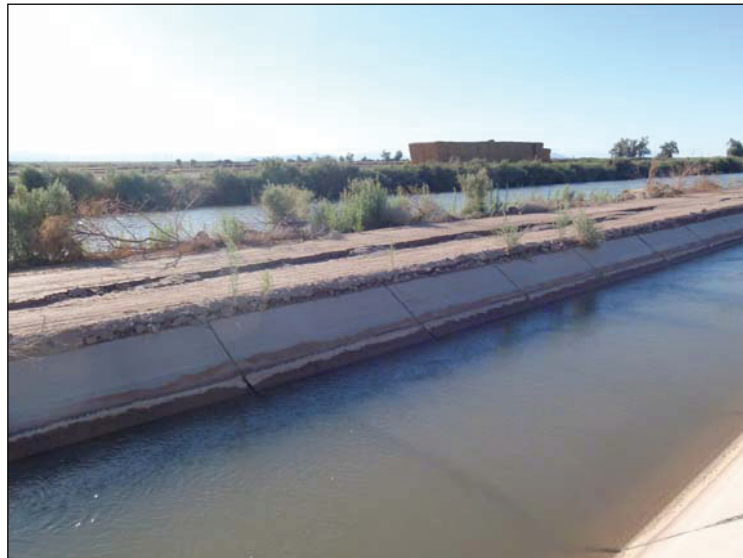
Figure 37. Lateral spread ground failure in a strip of fill separating the Westside Main Canal (background) from Wormwood Lateral (foreground) (C03). Photo by J. Tinsley, 4/7/10.
