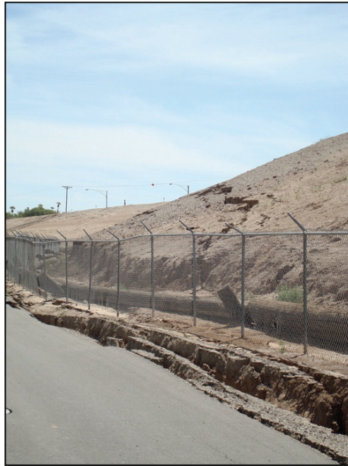
Figure 110. Liquefaction lateral spread and slump of waste water treatment plant access road (F04). A portion of the hill, probably fill, also experienced slumping. View to the southeast. Photo by T. McCrink, 4/10/10.
