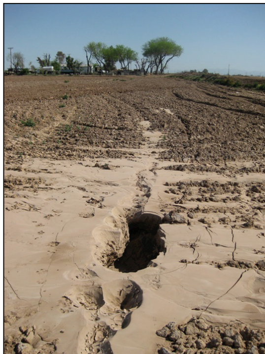
Figure 75. Large sand boil that formed along a fissure on the east side of the Rosita Canal (C56). The sand boil has an unusually large crater and the concentric cracks suggest subsequent caving. View to the south; the Rosita Canal is to the right of the picture. Photo by C. Pridmore, 4/11/10.
