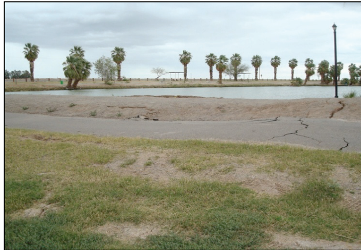
Figure 101. View of the south end of the Sunbeam Lake Dam crest, looking northeast (F02). Photo was taken 8 days after the earthquake. Transverse crack on the crest is larger and new cracks parallel to it are now visible. Cracks in asphalt are more pronounced and several newly visible cracks extend into the lawn area. The continued deformation may be the result of a week of strong aftershocks. Photo by T. McCrink, 4/12/10.
