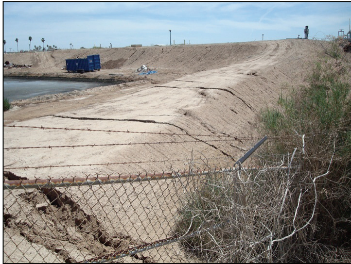
Figure 114. Lateral spread fissures extending through sludge drying ponds on the west side of the waste water treatment plant (F04). Fissure in the foreground is extensional and those in the middle of the picture show vertical displacement on the order of 2 to 5 cm. View to the southeast. Photo by T. McCrink, 4/10/10.
