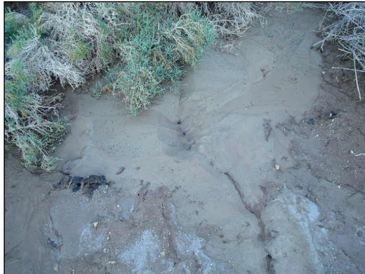
Figure 13. Vented sand in the marshy area east of the north approach fill to the Drew Road Bridge (R07). Lateral spreading damage to the road occurred immediately west. Photo by T. McCrink, 4/8/10.
