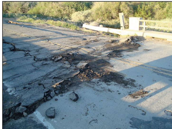
Figure 15. Battered asphalt on the north side of the concrete Drew Road Bridge structure (R07). Similar deformation was found on the south side as well. View to the northeast. Photo by T. McCrink, 4/8/10.
