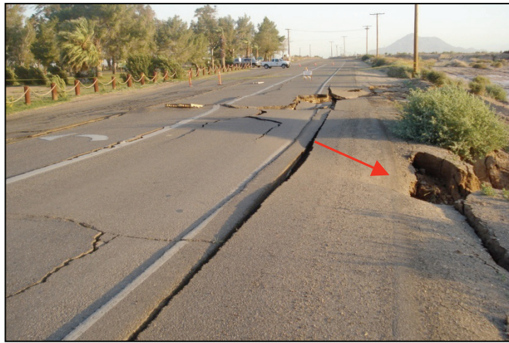
Figure 98. Liquefaction-related settlement and lateral spreading of Drew Road, immediately west of Sunbeam Lake Dam (R12). View is toward the south with El Centinela Peak in the distance. An eyewitness reported water geysering out of the pavement during the earthquake. Outlet pipes from Sunbeam Lake and from a large irrigation drain enter the stream to the right of the prominent slump in the center-right of the photo, indicated by the arrow. Both apparently were damaged by liquefaction. Photo taken 4/4/10; courtesy of the Imperial County Planning and Development Services Department.
