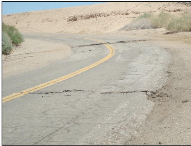
Figure 12. Possible liquefaction-related settlement in fill underlying Nichols Road, northeast of the New River (R06). Upper fissure had about 5 cm vertical displacement with extension in the asphalt, whereas the lower fissure had little vertical displacement but showed compression in the asphalt. Road-parallel fissures were observed in the fill embankment to the right of this photo. Photo by T. McCrink, 4/9/10.
