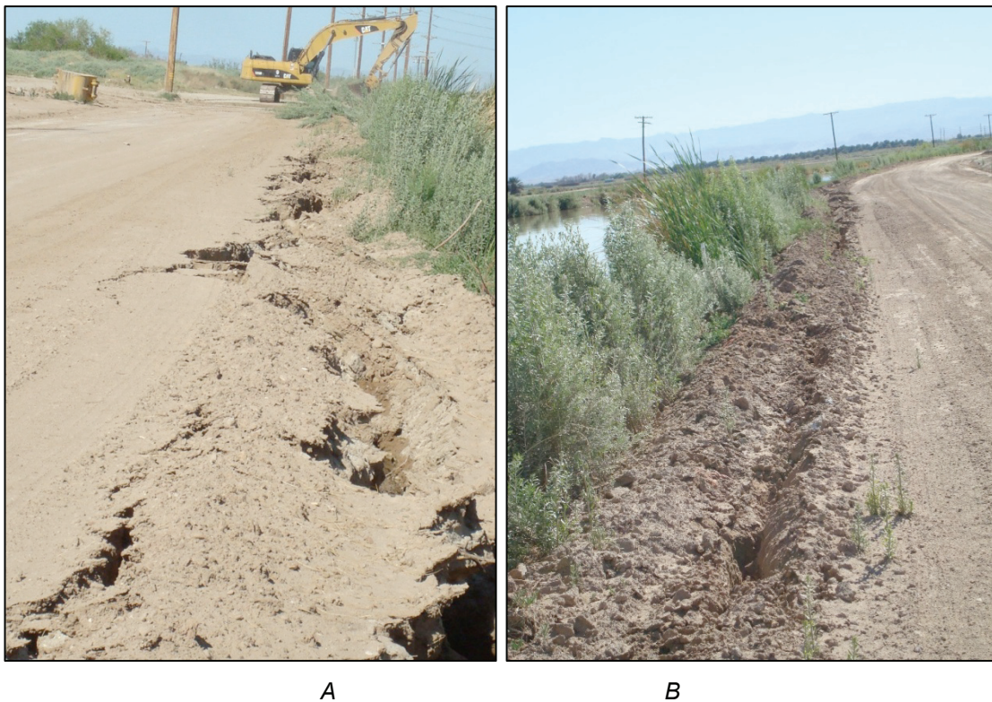
Figure 55. Failure of the Westside Main Canal west bank south of the Fillaree diversion structure (C51). A , View to northeast; excavator in the background is making repairs. B , View to the southwest of the same bank failure. Fractures end where the levee road turns to the right. Vegetation along the canal bank is tilted towards the channel and displaced tens of centimeters. Photos by T. McCrink, 4/8/2010.
