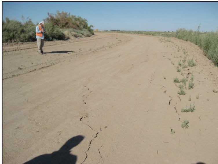
Figure 54. Set of three arcuate fractures across the full width of the levee on the west side of the Westside Main Canal (C44). Displacements amounted to a few millimeters, and the fracture set extended about 28 m along the Westside Main Canal. The last set of fractures is at the toes of the geologist on the left. Although no vented materials were observed, the morphology of the failure is consistent with the type of deformation produced by liquefaction. Photo by C. Pridmore, 4/8/10.
