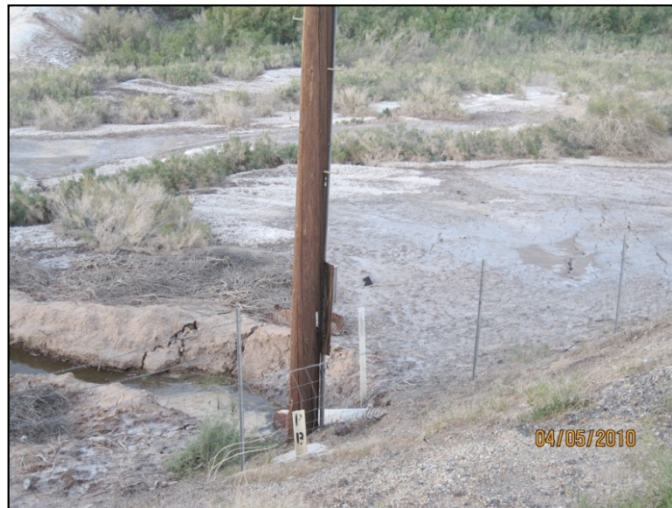
Figure 19. Lateral spread fissures and vented sand north of Interstate Highway 8 on the east bank of the New River (R08). These liquefaction features were only 50 m or less from the fill failure and pavement fractures shown in the previous figures, and they strongly suggest that liquefaction is responsible for the deformation of the highway. Photo by E. Seyhan, 4/5/10.
