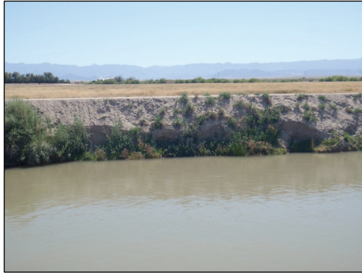
Figure 53. View to the west showing shallow slumping of the Westside Main Canal wall that dropped vegetation into the canal and oversteepened the canal-side face of the levee (C36). This stretch of slumping extended for 100 m. Photo by J. Tinsley, 4/7/10.
