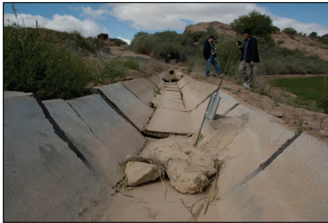
Figure 10. Effects of lateral spreading on the small irrigation canal adjacent to Lyons Road (R06). Photo by S. Brandenburg, 4/5/10.
