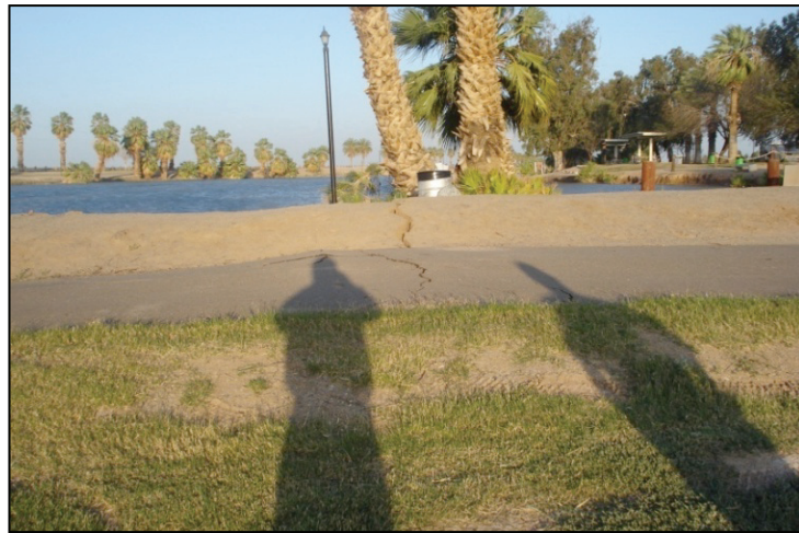
Figure 100. View of the south end of the Sunbeam Lake Dam crest, looking east (F02). Photo was taken soon after the earthquake. Dam crest to the left has dropped 15 to 30 cm relative to the area to the right of the large crack in the center of the photo. Photo courtesy of Imperial County Planning and Development Services Department.
