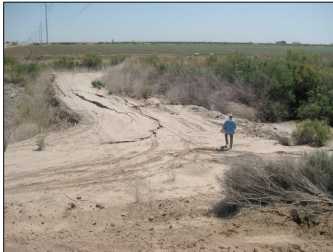
Figure 78. View to the east across Greeson Drain at liquefaction lateral spread fissures in the access road fill prism (D03). The full width of the road fill settled and the northern two-thirds spread to the north. Photo by C. Pridmore, 4/9/10.
