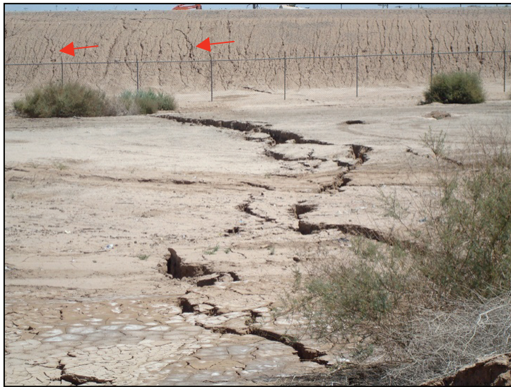
Figure 116. Liquefaction lateral spread fissures extending across New River flood plain into pond embankments on the west side of the Waste Water Treatment Plant (F04). Arrows point to fissures in the embankment. At the time of the California Geological Survey visit, a track-mounted excavator (orange machine arm in the top center of this photo) was making repairs in the center of the plant at a point suspiciously in line with these fissures. View to the east from the large scarp shown in figure 115. Photo by T. McCrink, 4/10/10.
