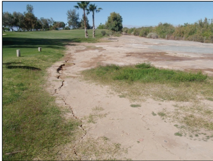
Figure 87. Liquefaction lateral spread west of the Rio Bend RV Park (D11). Golf course on the left and New River active channel is at the right immediately beyond the line of riparian vegetation. A horizontal extension of about 15 cm was measured. Wet vented sand, dark brown in the photo, was observed here, 3 days after the mainshock. Photo by J. Tinsley, 4/7/10.
