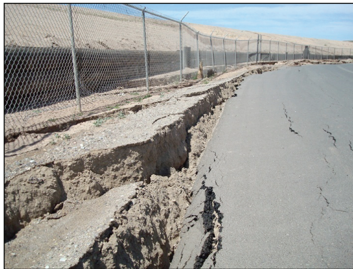
Figure 109. Liquefaction lateral spread and slump of waste water treatment plant access road (F04). A matching but smaller uphill-facing scarp on the other side of the road indicates that the soil under the pavement settled and rotated. Geotextile was observed in exposed road base, which may have helped keep pavement from experiencing the intensity of fissuring observed on the sides of the road. View to the west. Photo by T. McCrink, 4/10/10.
