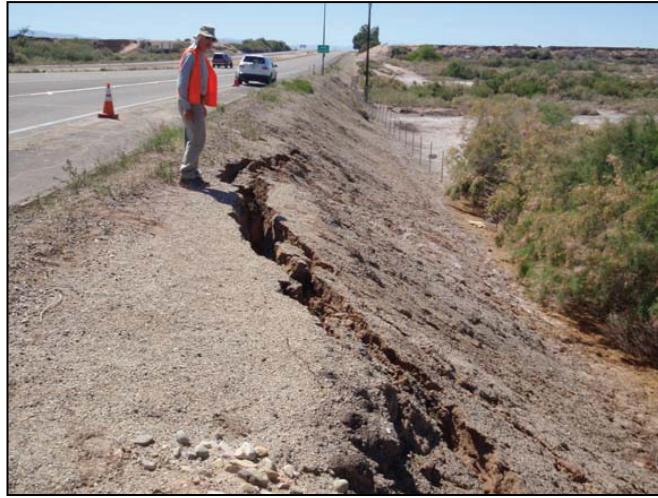
Figure 18. Extensional fractures and fill failure on the north side of Interstate Highway 8 and east bank floodplain of the New River, just north of the extensional fractures shown in figure 17 (R08). All deformation here inferred to be due to liquefaction on the basis of the presence of lateral spread fissures and vented sand on the New River flood plain 50 m or less to the west. Photo by J. Tinsley, 4/7/10.
