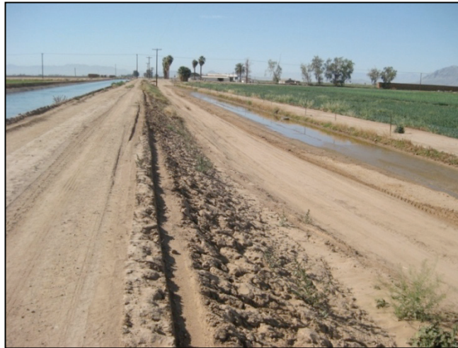
Figure 67. View to the southwest along Nichols Road showing ponded water in a low lying area along Nichols Road (C40). This area is located approximately 150 m north of McCabe Road, which is marked by the trees in the background. Soils on the outer levee side that have not been disturbed by postearthquake traffic show erosion caused by water flow. Photo by C. Pridmore, 4/11/10.
