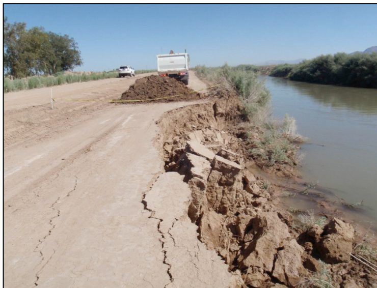
Figure 52. Probable liquefaction-related lateral spread slump into the Westside Main Canal (C35). Soil was being imported on 4/7/10 prior to repairs. Photo by J. Tinsley, 4/7/10.
