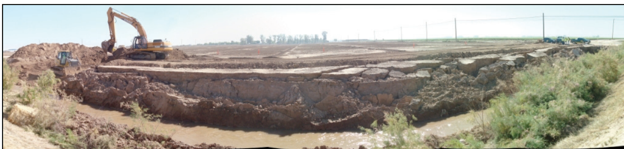
Figure 89. Panoramic view of the lateral spread at Evan Hewes Highway (on the right along the line of telephone poles) and Rice Drain No. 3 (foreground) (D12). Repairs underway on the left consist of excavation and replacement of the levee materials. Photos by T. McCrink, 4/9/10.
