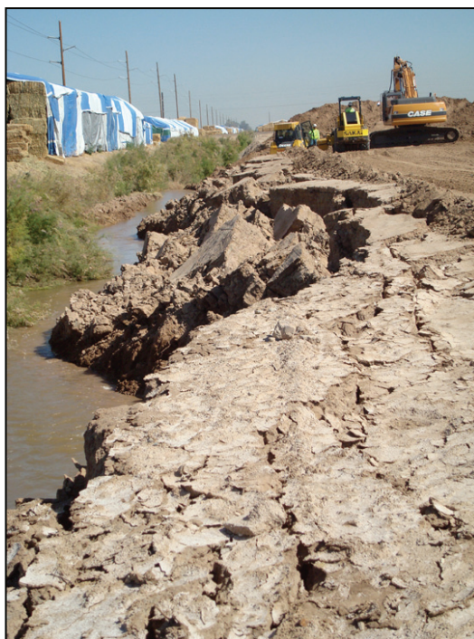
Figure 90. View looking north at the lateral spread into the Rice No. 3 Drain (D12). Owner of the agricultural field reported that the salt cedar bushes now on the west bank were on the east bank before the earthquake. Photo by T. McCrink, 4/9/10.
