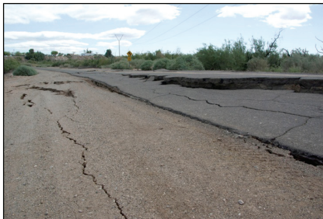
Figure 9. Settlement of Lyons Road pavement and north shoulder owing to lateral spreading within the zone of liquefaction deformation shown in the preceding photo (R06). Photo by S. Brandenburg, 4/5/10.
