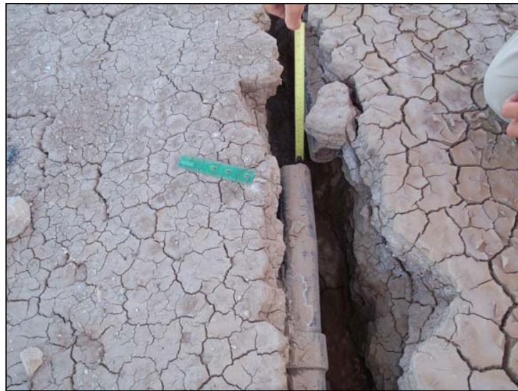
Figure 35. Liquefaction-induced extensional fracture near the junction of the Westside Main and All American canals (C01). Exposed pipe or conduit offset 70 mm. Vented sand partly fills fracture underneath the offset pipe. Spreading vector was towards the Westside Main Canal. Photo by J. Tinsley, 4/6/10.
