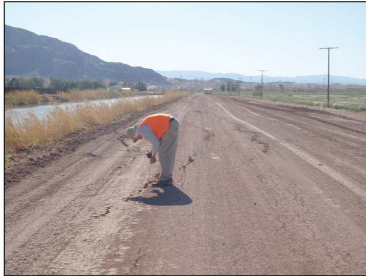
Figure 57. View looking west across the westernmost set of arcuate extensional fractures that deformed the north bank of All American Canal near Pullman Road (C02). This failure is 58 m long and open fractures were plumbed to depths of about 135 cm. Differential settlement is about 85 mm and total extension across apparent lateral spread is greater than 12 cm. No vented materials noted. Building in the distance marks the end of the All American Canal and the beginning of the Westside Main Canal. Photo by J. Tinsley, 4/6/10.
