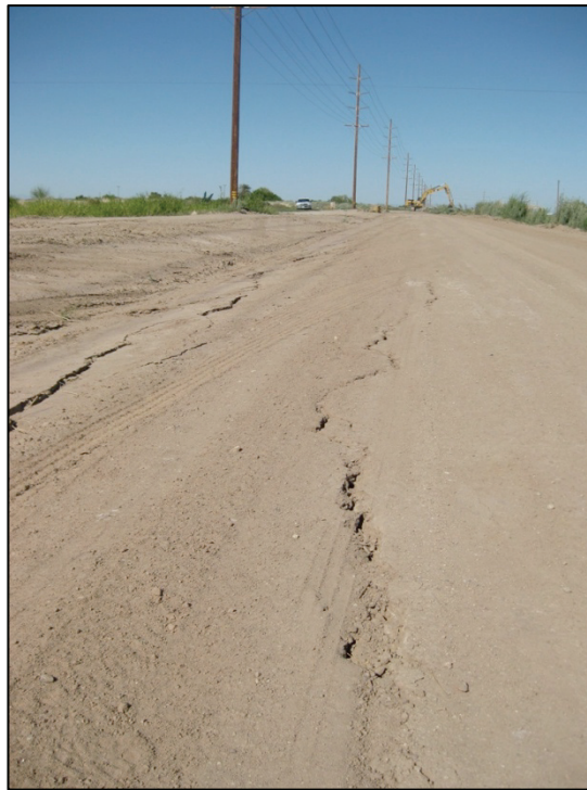
Figure 56. View to the northeast of fractures running through the outer edge of the Westside Main Canal levee road (C51). Extensional and vertical displacements are one to several centimeters with displacement downward and toward the canal. Photo by C. Pridmore, 4/8/10.
