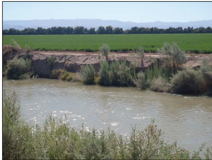
Figure 51. View of the west side of Westside Main Canal, showing recent bank failure and slumping of vegetation-bearing soil into the canal (C34). These shallow bank failures were extremely common on both sides of the Westside Main Canal throughout the examined reaches. Photo by J. Tinsley, 4/7/10.
