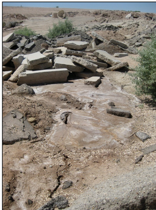
Figure 111. Liquefaction vented sand and related cracking in nonengineered fill adjacent to the Treatment Plant access road (F04). Access road is at the base of the hill in the distance and the airport is just beyond. View to the southwest. Photo by C. Pridmore, 4/10/10.
