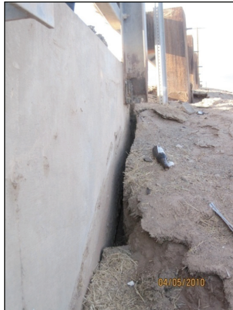
Figure 6. Approximately 5 cm separation of embankment soil from the concrete abutment at the Brockman Road Bridge over the New River (R05). Photo by E. Seyhan, 4/5/10.
