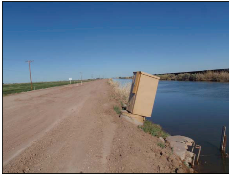
Figure 34. Former stage gauge stilling tower tilted from vertical at the Westside Main Canal; associated structures visible to the right of the tower were also tilted from plumb and damaged (C01). No vented materials visible locally. Photo by J. Tinsley, 4/6/10.
