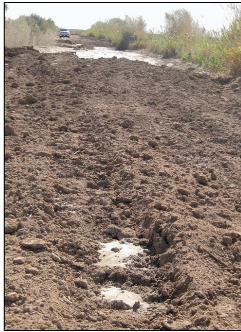
Figure 86. Vented sand (bottom center) on a recently regraded levee next to Fig Lagoon, indicating that liquefaction of saturated soils continued to occur during aftershocks (D10). Fig Lagoon lies to the right of the vegetation in the upper right. Wet area between graded material in the foreground and vehicle in the background is where lateral spreading and overtopping of lake water occurred (figs. 80 and 81). Photo by C. Pridmore, 4/10/10.
