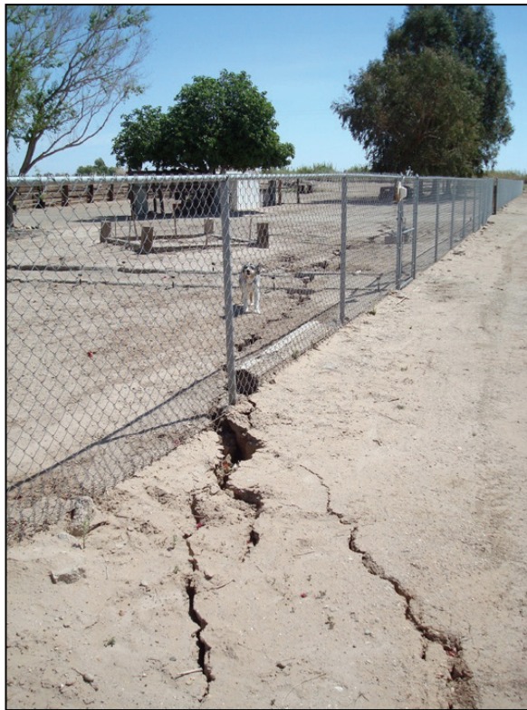
Figure 72. An arcuate lateral spreading crack running through a fenced yard on the north side of the Rosita Canal, northeast of the intersection of East Alamo and Bell roads (C56). Vented sand was found in several areas on both sides and filled some parts of the crack. The levee road, just to the right of the picture, had recently been graded, obliterating any liquefaction features that may have existed. View to the east. Photo by T. McCrink, 4/11/10.
