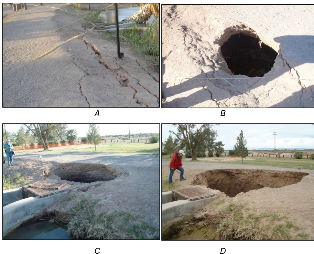
Figure 102. Time sequence photographs of a sinkhole that formed on the Sunbeam Lake Dam (F02). A , The dam crest and outlet weir on the day of the earthquake. Photo courtesy of Imperial County Planning and Development Services Department. B , Early stage of sinkhole formation on the morning of 4/7/2010; the person whose shadow partly covers the sinkhole is standing on the outlet weir. Photo by J. Tinsley. C , Sinkhole on the evening of 4/8/2010. Photo by T. McCrink. D , Sinkhole on 4/12. Photo by T. McCrink.
