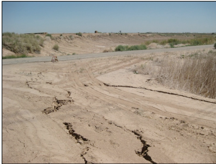
Figure 77. View looking northeast across Lyons Road and down Greeson Drain (D03). The culvert under Lyons Road is located to the right of this photo but the settlement in fill in the foreground appears to continue beneath Lyons Road. North of Lyons Road the drain bottom, slopes, and upper edges have all recently been regraded. Photo by C. Pridmore, 4/9/10.
