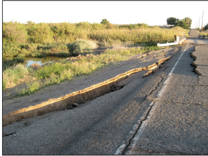
Figure 14. Lateral spreading of the north approach fill to the Drew Road Bridge (R07). Vented sand shown in figure 13 is immediately left of this photo. View to the south. Photo by T. McCrink, 4/8/10.
