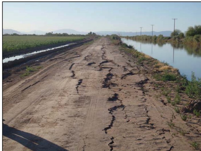
Figure 45. View to the northwest along the western levee of the Westside Main Canal showing large lateral spread ground failure that spanned the entire width of the levee (C25). The ground failure extended about 200 m along the levee, and the small in-facing scarplets indicate that the levee mass sank differentially into a liquefied substrate. Photo by J. Tinsley, 4/7/10.
