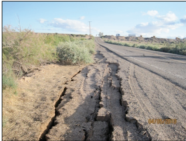
Figure 7. Ground cracking, settlement, and lateral deformation along the south approach to the Brockman Road Bridge crossing the New River (R05). Photo by E. Seyhan on 4/5/10.
