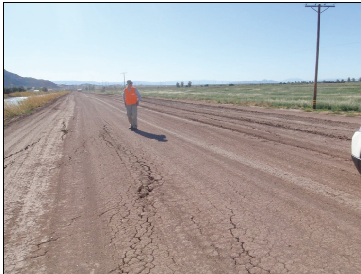
Figure 58. Wide-angle perspective image showing an incipient extensional failure that extends nearly across the entire width of the north embankment of the All American Canal near Pullman Road (C02). Total length of southward-extensional deformation exceeds 30 m. Liquefaction unconfirmed as no liquefied materials were vented. In-facing scarps indicate differential settlement involving the highest parts of the earthen levee. This pattern of deformation is consistent with liquefaction. Photo by J. Tinsley, 4/6/10.
