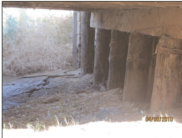
Figure 4. Lateral spread ground cracking on the north bank of Greeson Drain beneath the Brockman Road Bridge (R02). Photo by E. Seyhan, 4/5/10.
