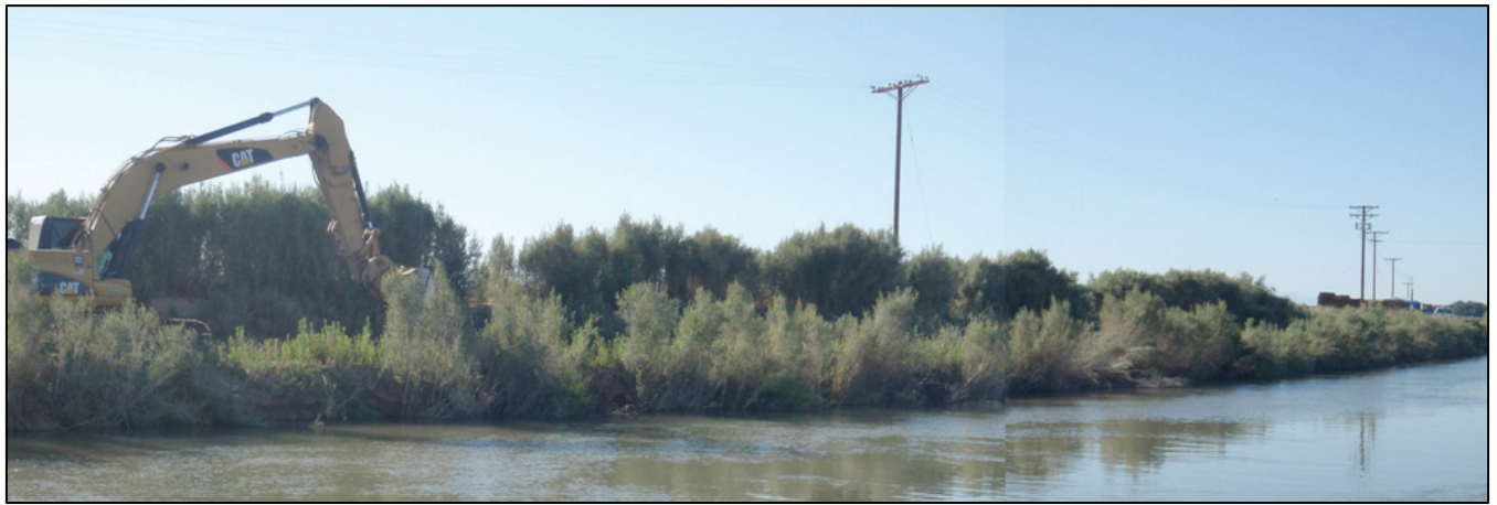
Figure 43. Ongoing repairs to the west bank of the Westside Main Canal on 4/7/10 (C15). Tilted and submerged vegetation indicate marked displacement of the levee bank. Photos by J. Tinsley, 4/7/10.
