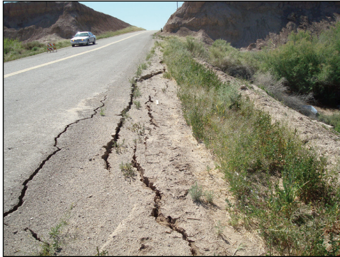
Figure 23. Lateral spreading fissures in approach fill on the northwest side of the Worthington Road Bridge over the New River (R18). Similar fissures were observed on the south side, but no vented sand was found. View is to the west. Photo by T. McCrink, 4/8/10.
