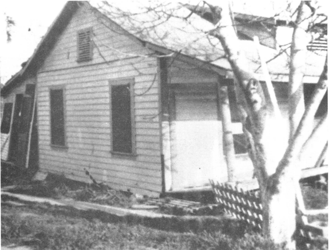
Photograph 2. House in the Long Beach-Compton area, displaced off its foundation in the 1933 earthquake. Photo by Olaf P. Jenkins.
