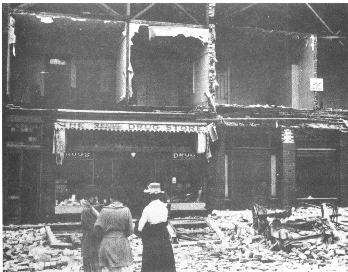
Photograph 3. Buildings damaged during 1920 Inglewood earthquake on western side of Commercial Street (now Brea Avenue) in Inglewood. Photo reproduced from Plate 8 of Taber (1920).
