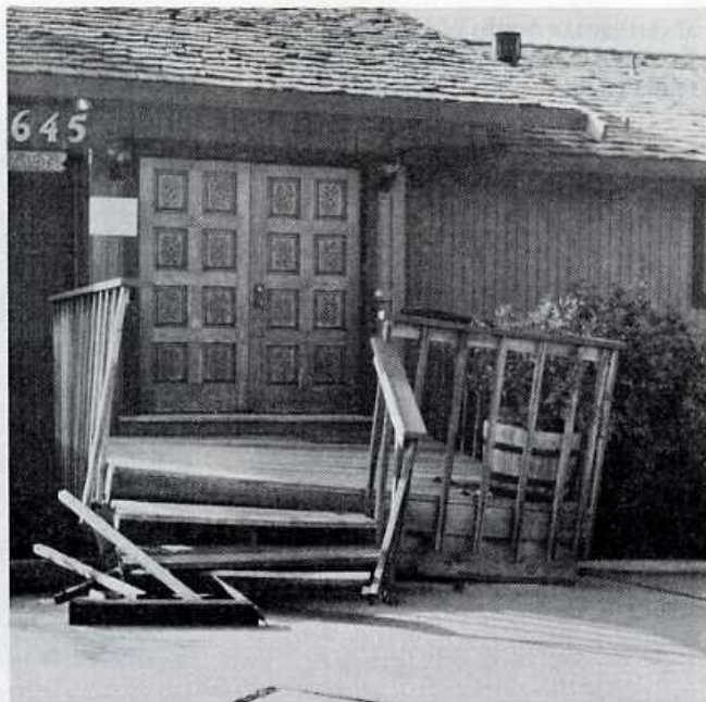
Structural damage, Morgan Hill.
