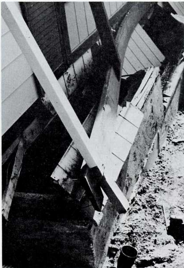
Structural damage, Morgan Hill.
