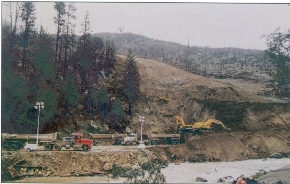
Photo 5. Caterpillar tractors push landslide debris downslope toward two sets of track-mounted loaders at the toe of Mill Creek landslide. The roadbed was found to be intact after 27 days of excavation. Photo by Robert H. Sydnor.
