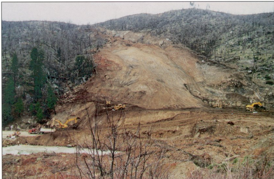
Photo 4. Heavy equipment removing an estimated 250,000 to 300,000 cubic yards (190,000-230,000 m 3 ). Photo by Robert H. Sydnor.
