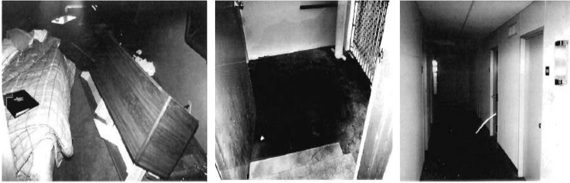
Fig.14: Non-structural damage during Northridge earthquake
