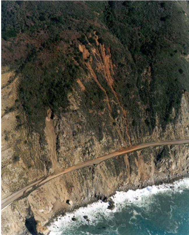
Figure 5. Cut slopes south of Limekiln State Park were subject to small shallow landslides in 1998. These slides included debris slides from loose, slightly weathered rock, on the left, and debris flows from older, dark reddish brown colluvium, on the right. Photo by L. Highland. Caltrans.
