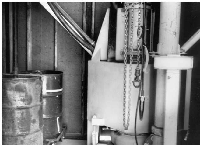
Photo 18. Pump and concentrate barrels located inside shed beneath spiral assembly.
