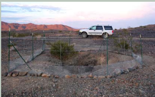
The Rusty Gold Mine in Riverside County following AMLU's construction of a fence around the open shaft.
