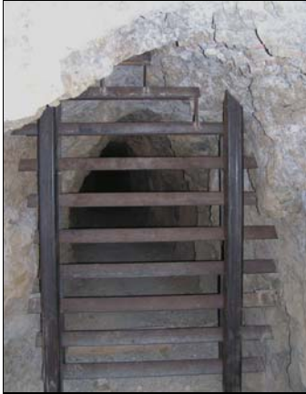
This bat gate, installed in an abandoned mine in San Bernardino County, allows bats to freely enter and leave the mine, but helps to ensure public safety.
