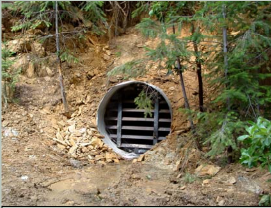
A culvert gate constructed at the Otter Creek Mine in El Dorado County.
