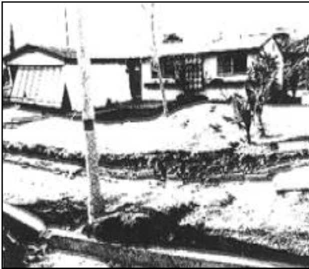
Photo 1. Single story wood frame houses usually stand up well to earthquake shaking. Even though fault rupture extends beneath this structure, it did not collapse during the 1971 San Fernando earthquake. The garage, however, with the large opening in the front, did yield to the horizontal shaking. Photo by R. Castle, courtesy of U.S. Geological Survey.
