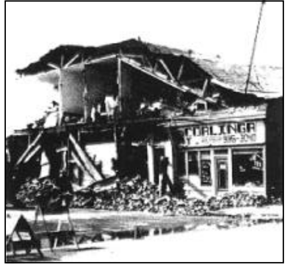
Photo 2. Masonry structures with little or no reinforcement, such as those in the Coalinga business district, usually sustain the greatest damage during an earthquake. Photo by James Stratta.
